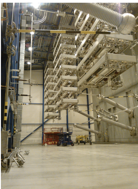
Valve towers are the heart of converter stations
