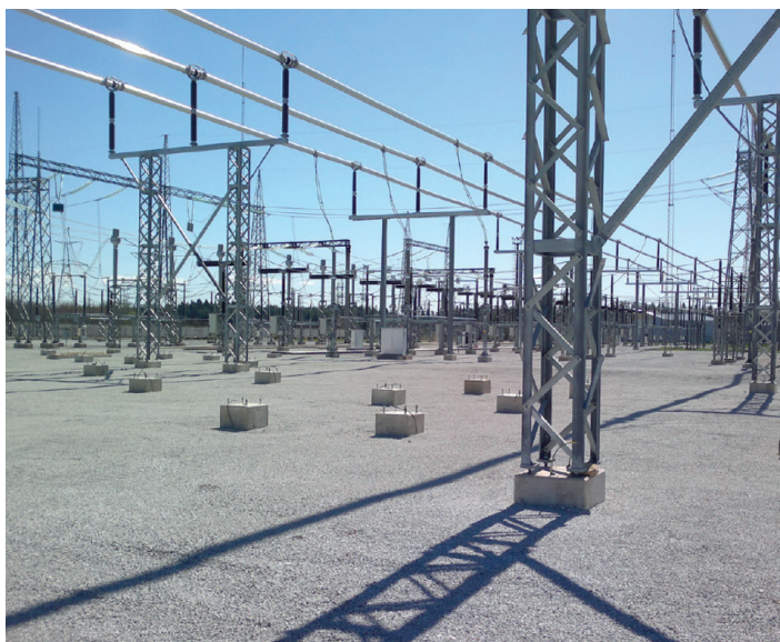
Püssi AC substation was renovated and extended for EstLink 2
