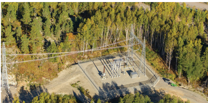
Transition from submarine cable to overhead line in Finland is made in Nikuviken station
