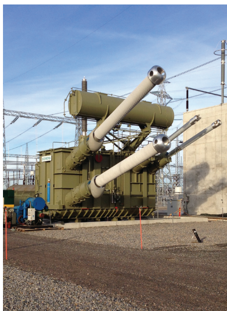
One phase three winding converter transformers are used in EstLink 2 project
