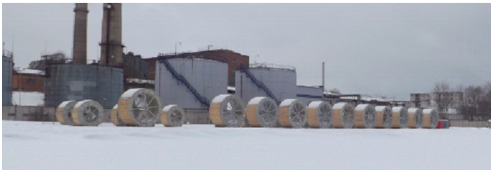
Land cable route preparation works in the Nordic climate were not an easy task
