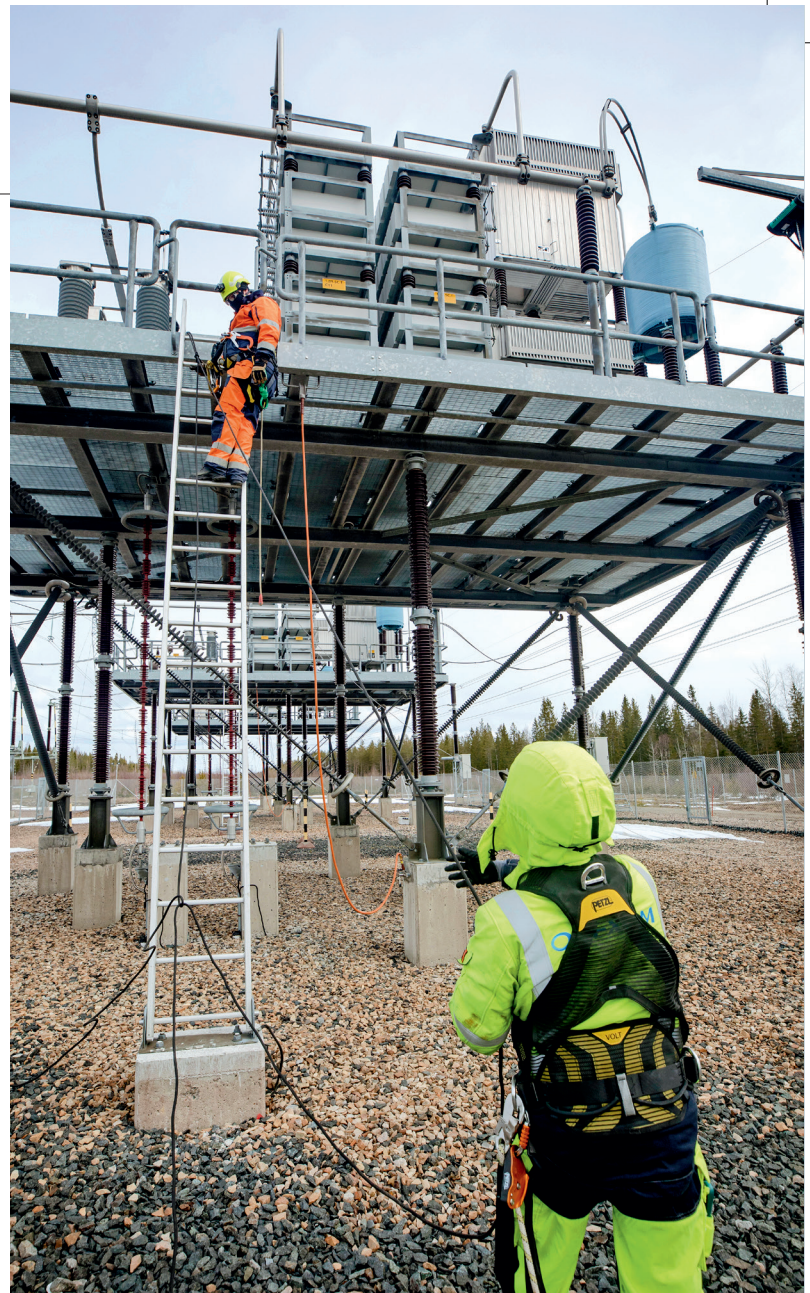
The structures at the Keminmaa substation are appropriate, but additional anchorage points are required for tasks such as getting off the ladder.
