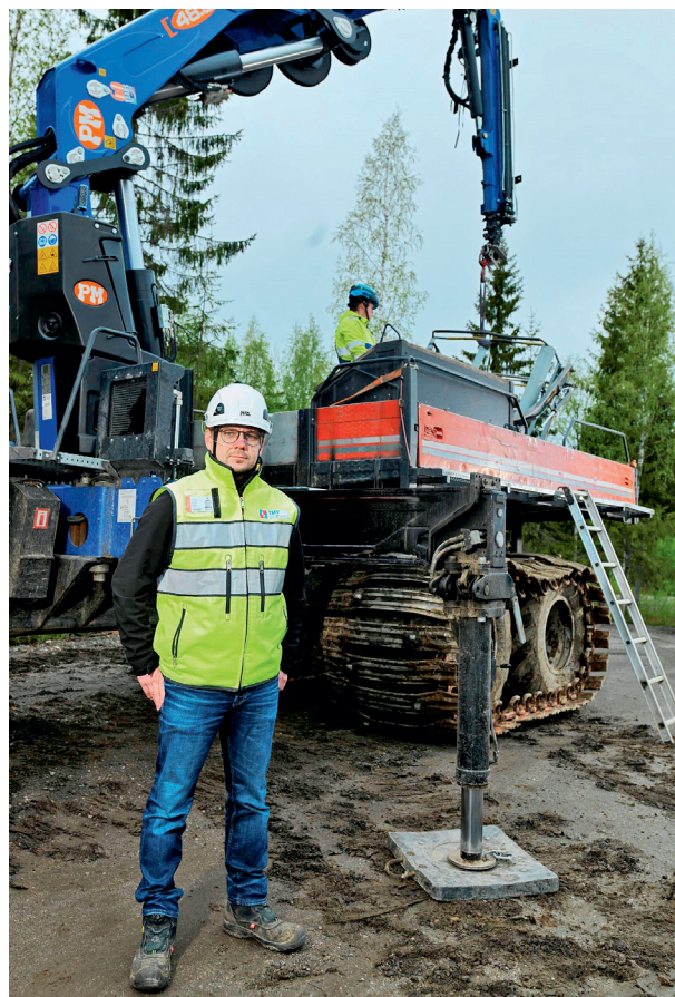
Jani Rintala, Project Manager from TMV Line, is satisfied with the changes made to the work machine to improve safety.
