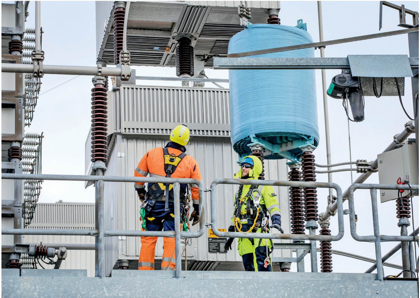
The trial climb of the Keminmaa substation involved climbing onto the platform of the series capacitor and working there.
