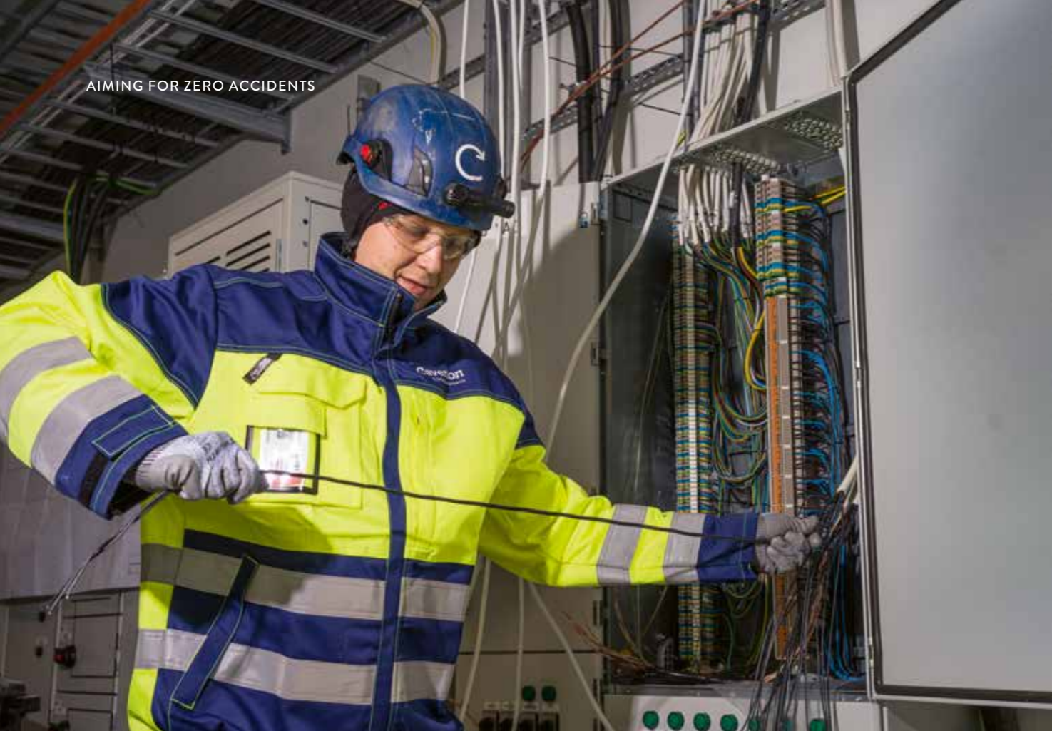
The Valkeus substation worksite met all of Fingrid's preventive safety targets last year.
