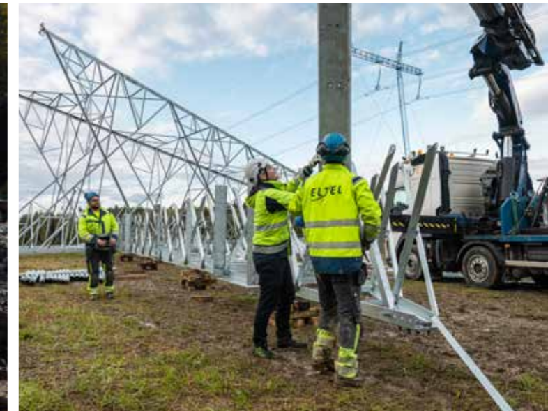
Ricards Andzans (left) and Jukka-Pekka Kivistö (centre) carry out a lift on a worksite.
