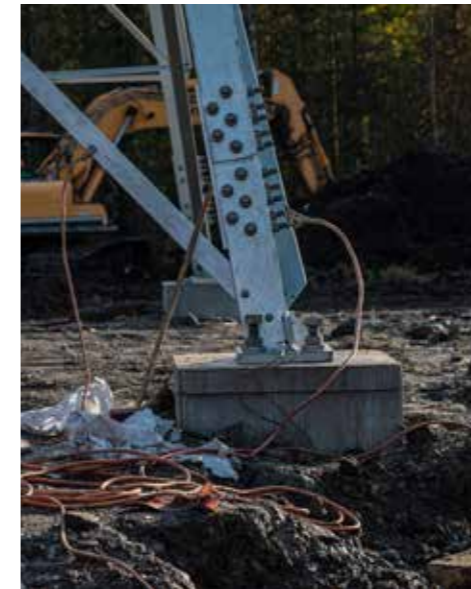
Cranes and other work machinery operating near the live line are earthed with care.
